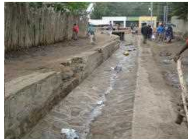
Improper drainage location
