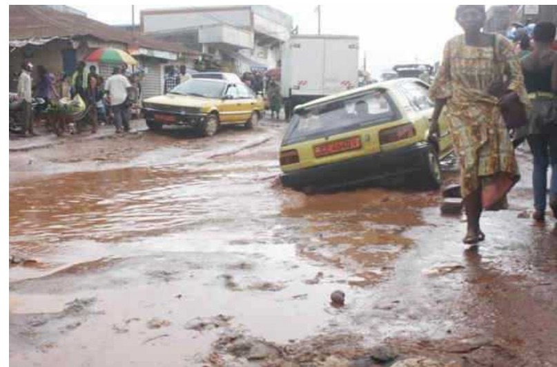
Dammaged road using by pedestrians,sellers, small and big vehicles
