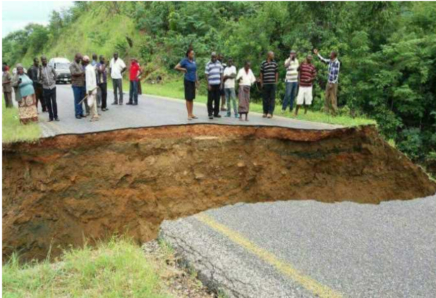
Collapse in RN 1 after heavy rain RN 1(大雨の後に崩壊)
