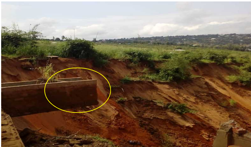
Slope failure, gutter suspended after heavy rain (Road Agency)
